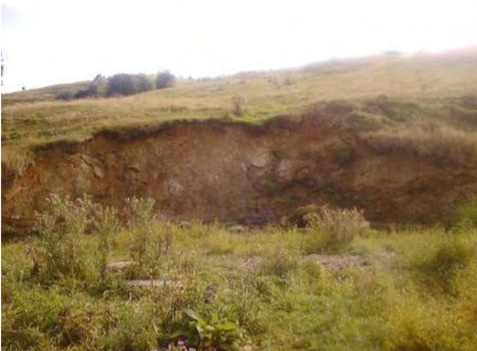
Figure 15: An example of slip erosion; coding and description. SI (A) o 15 x 3.5 m N: Slip, (active), outside, 15 m long, 3.5 m high, not protected.
