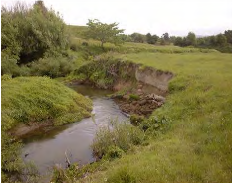
Figure 18: An example of slump erosion; coding and description. Sm (A) o 10 x 2 m N: Slump, (active), outside bend, 10 m long/2 m high, not protected.
