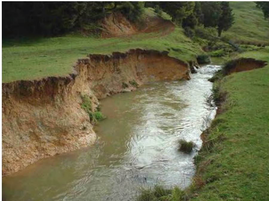
Figure 12: An example of scour erosion; coding and description. Sc (A) s 15 x 1.5 m N: Scour, (active), straight, 15 m long, 1.5 m high, not protected.
