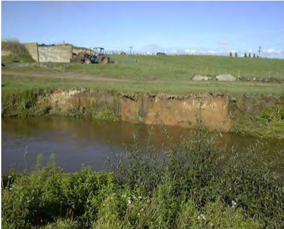
Figure 14: An example of active and unstable scour erosion; coding and description. Sc (U) o 5 x 1.5 m N and Sc (A) o 5 x 1.5 m N: Scour, (unstable), outside, 5 m long, 1.5 m high, not protected and scour, (active), outside, 5 m long, 1.5 m high, not protected.
