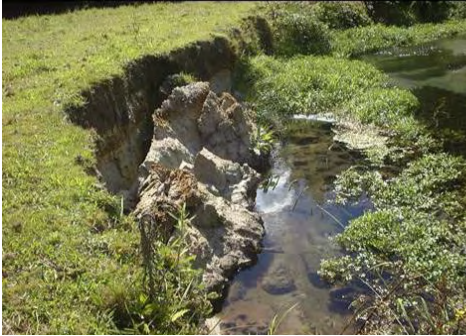
Figure 20: An example of slump erosion; coding and description. SI (A) o 6 x 1.5 m N: Slump, (active), outside, 6 m long, 1.5 m high, not protected.
